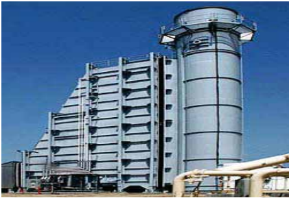
Contracted power generation
