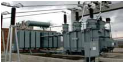
Regulated electricity distribution
